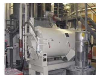
After: New Heating and Cooling Mixer vessels
